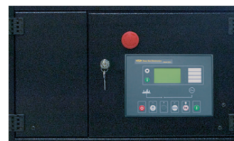
Deep Sea 7210 Control Panel
